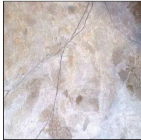
Granicrete cracked stone floor working with the cracks
